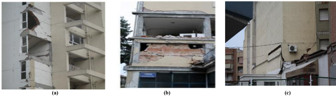
Fig. 1. Out-of-plane collapse of masonry infill walls observed during past earthquakes ;(a) Nepal earthquake, 2015 [1]; (b) Kermanshah earthquake, 2017 [2]; (c) Spain earthquake, 2011 [3].
